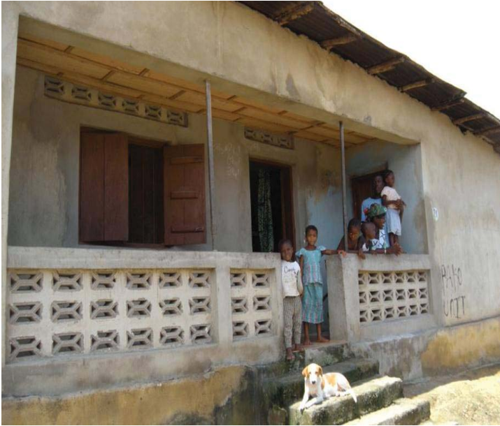
Renovations have begun on an interim home for child victims of labor or trafficking. The home is about 10 minutes from the CRC.
