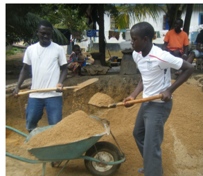
CRC children building a new home for a needy family in their community.
